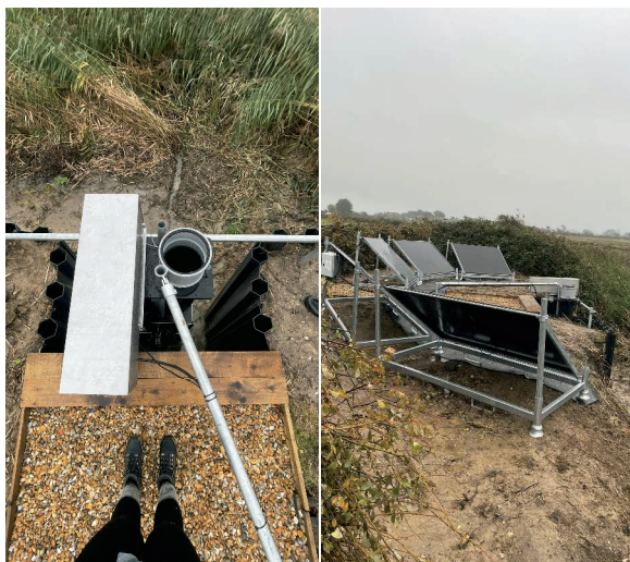
The Solar Pump showing the pump mechanism and the solar panels, hidden behind a willow screen beautifully made by volunteers
